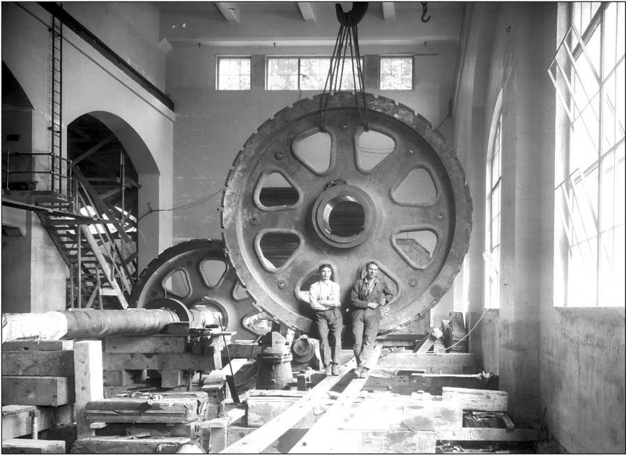
British Columbia was industrializing rapidly in the first years of the twentieth century. The Buntzen Lake Power House No. 2 (shown under construction in 1913) was among the new industrial projects. City of Vancouver Archives LGN832.
